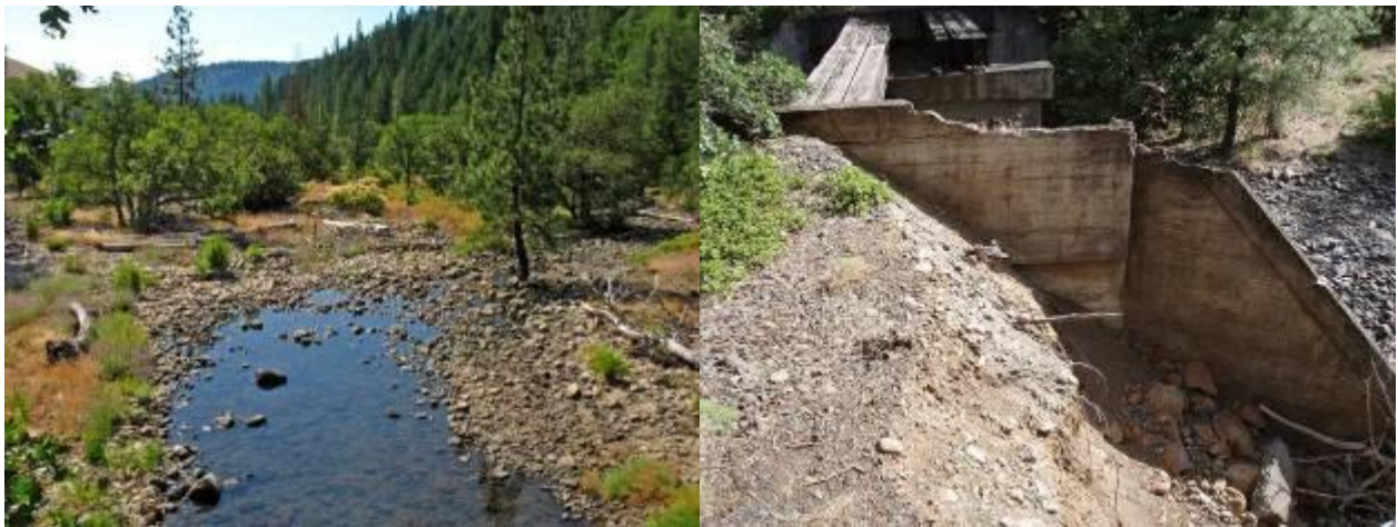
Figure 16. Tail-out of scour pool created by trestle (left) and embankment erosion (right).
